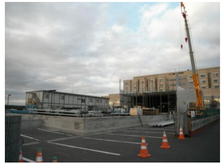
Construction under way in the former parking lot of Ishinomaki Red Cross Hospital. ©JRCS
